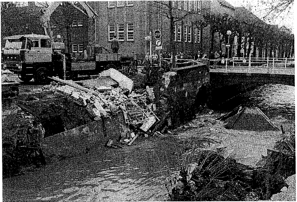
Photo 9.2 A few hours after the flood peak at the same location as on Photo 9.1: the electricity station and the sheet-pilings are devastated.
